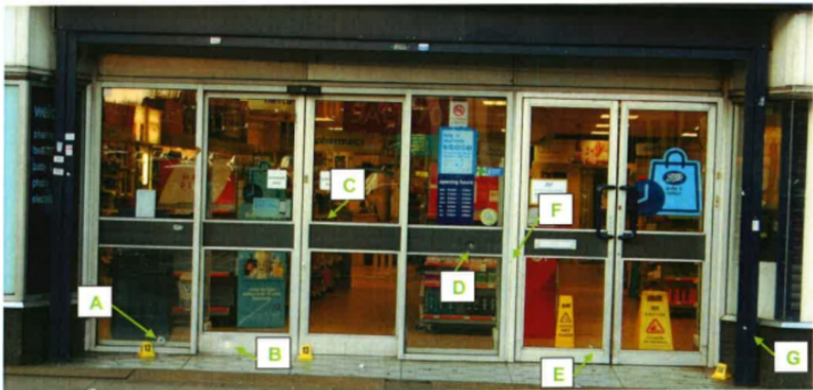
Image 6: entrance of Boots with damage sites identified
